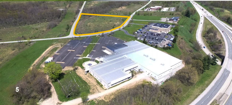
Construction of a new 20,604 sf test pool facility and a 30,500 sf expansion of the Advanced Acoustic Concepts (AAC) building in the University Business Park, North Union Township.
