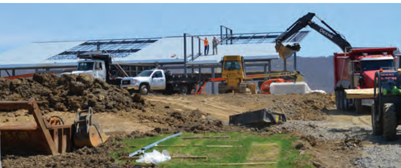
Sleighter Engineering's building currently under construction at the University Business Park, North Union Twp.
